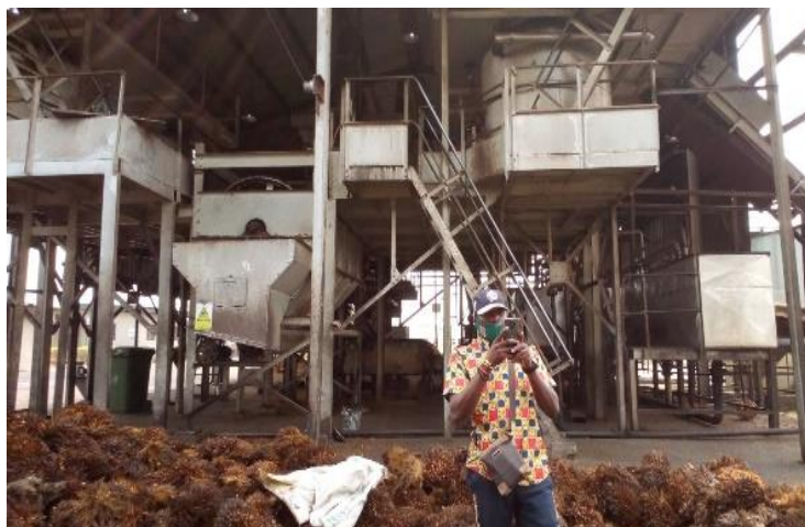
Figure 6: JB Farms Functioning Palm Fruit Processing Plant
