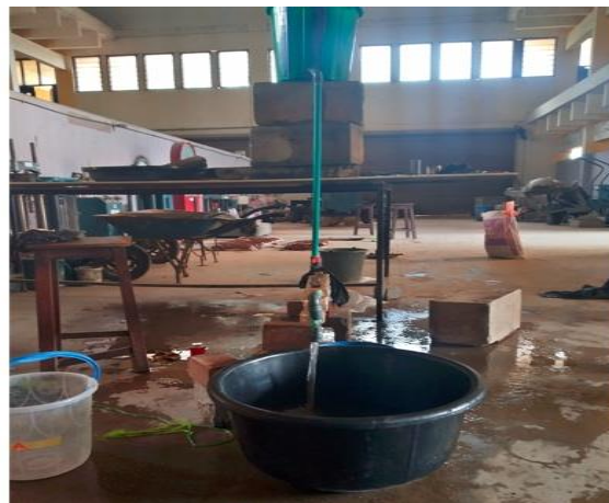
Figure 2: Pictorial view of the water tank connected to the magnetic water treatment unit
