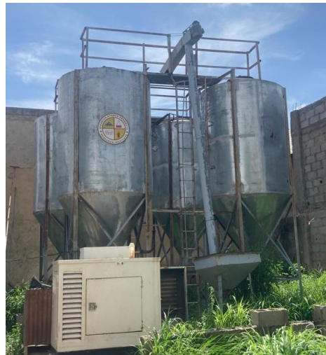
Figure 1. Inert atmosphere silo installed at the Dawanau International Grain Market, Kano
